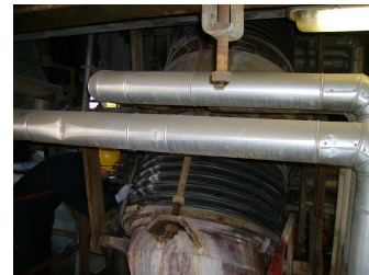
Spring hanger removed without block EJ
